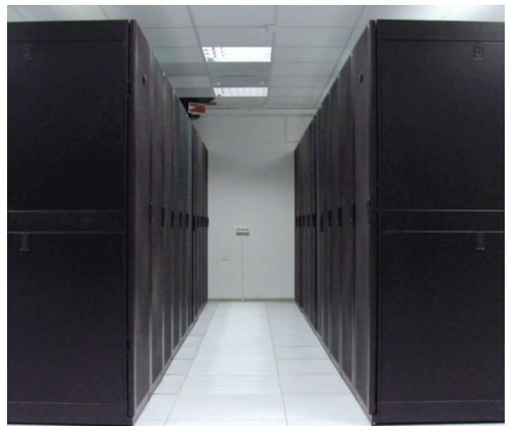
EPAM Systems Data Center
