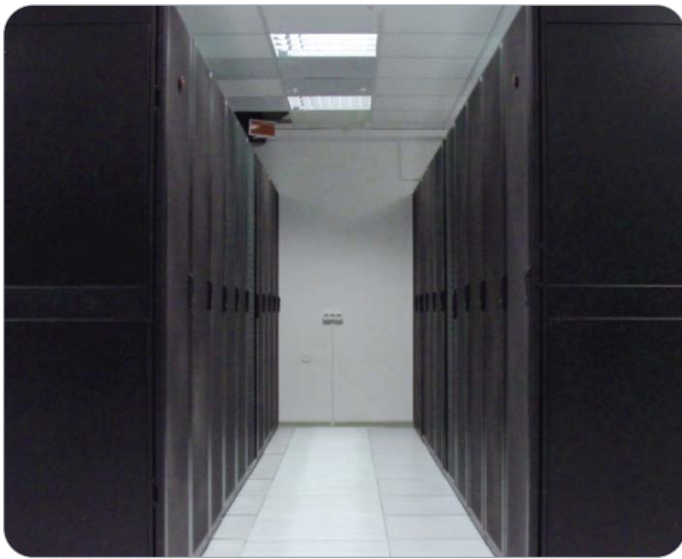
EPAM Systems – Rechenzentrum
