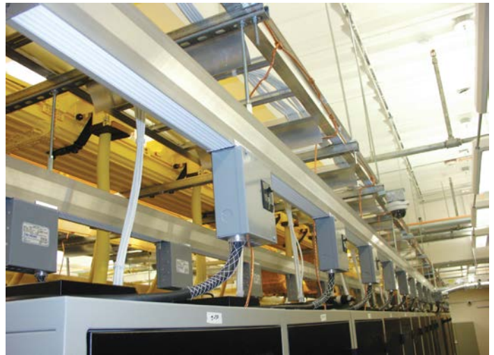
Power can be accessed at any location along the busway system, eliminating the need for power boards, long runs of wire and expensive installation costs.
