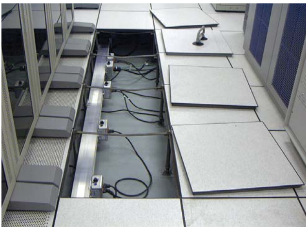
A clean, organized power busway system simplifies power distribution and can lower HVAC costs.
